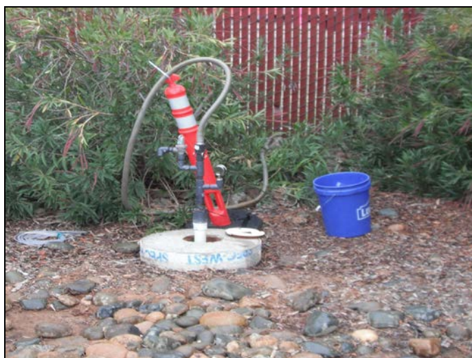
Site SS023 ISCO injection well.
