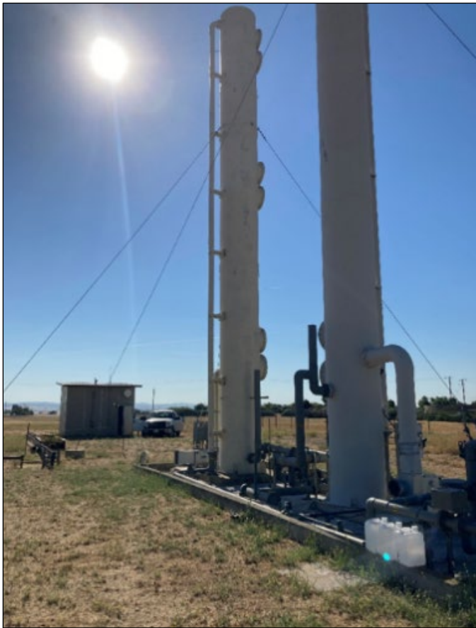
Extraction of groundwater by the CG044-013 Groundwater Treatment System.
