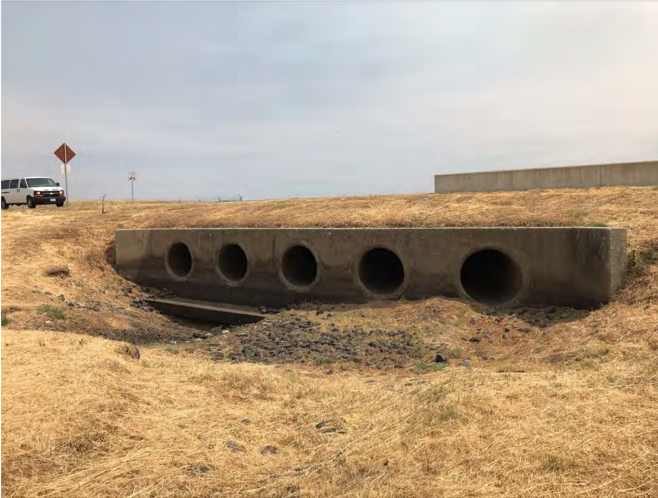
Photograph 3: Activity 14 – Repair Road and Culvert at Doolittle Gate. Photo of Reeds Creek culverts from west side of Doolittle Drive looking northeast, taken August 17, 2021.
