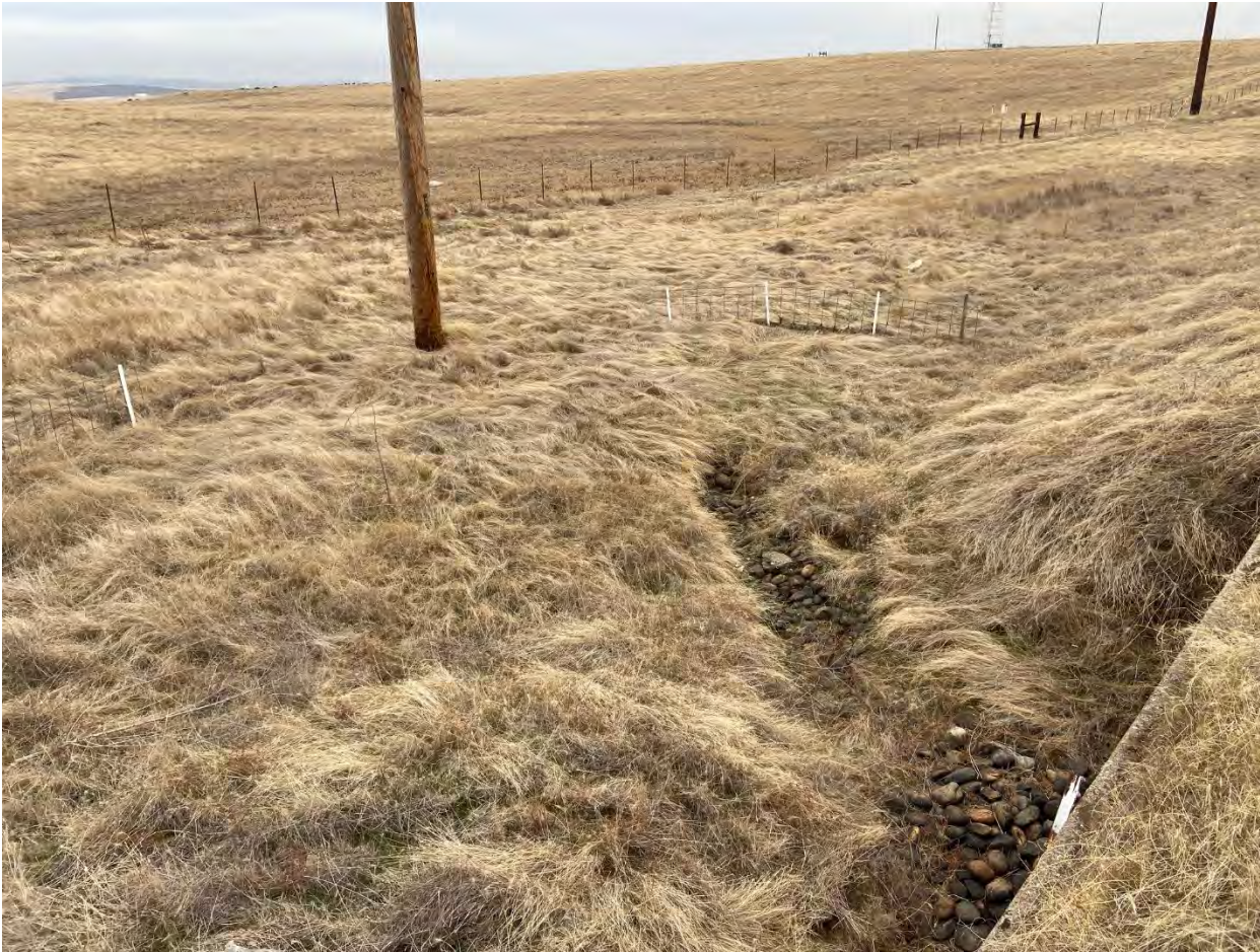
Photograph 4: Location of Activity 15 – Repair Storm Drainage, B1029. Drainage that feeds into the eastern side of the B1029 storm drainage system. Photo taken August 17, 2021, from Doolittle Road looking east.
